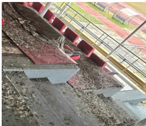
Figure 3 Stands covered with pigeon droppings
