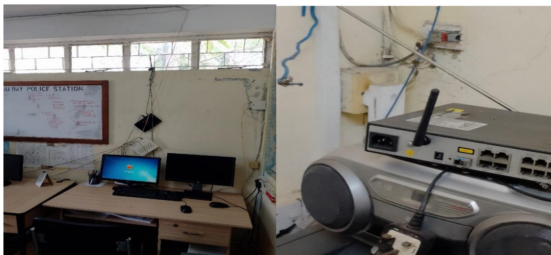
Figure 4 Poor Wiring and Cabling works at Baie du Tombeau Police Station
