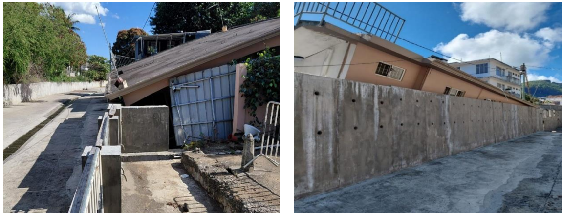
Figure 13 Damaged House at Tranquebar
