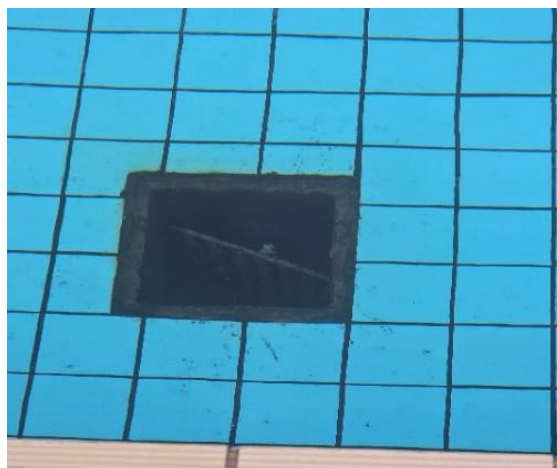
Figure 10 Rusted grill in the pool
