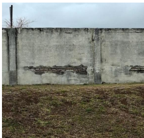
Figure 8 Damaged Safety walls
