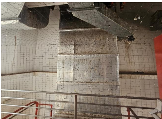
Figure 19 Droppings and nests of pigeons on ductwork
