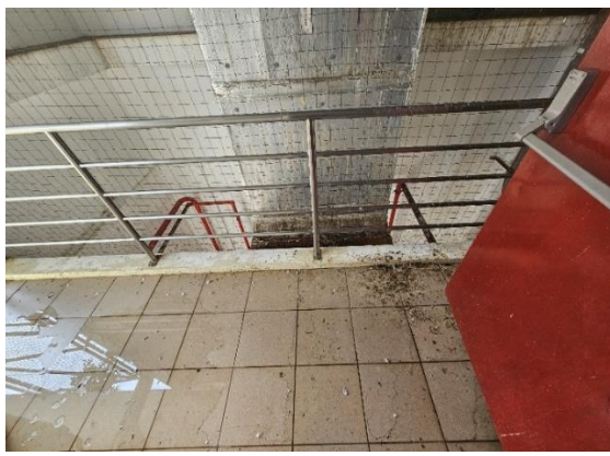
Figure 20 Droppings of pigeons at balcony of Chemistry Laboratory
