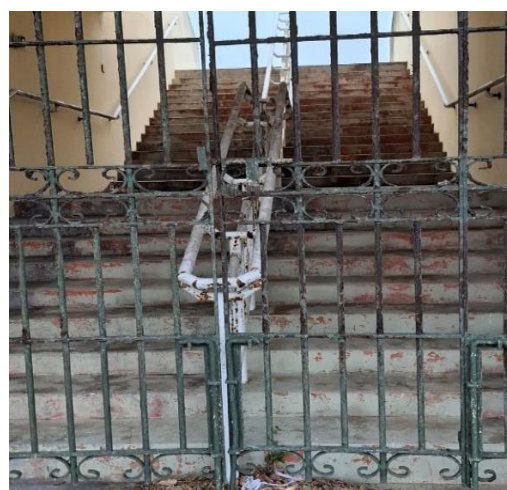
Figure 6 Gate and handrail leading inside stadium in rusted state
