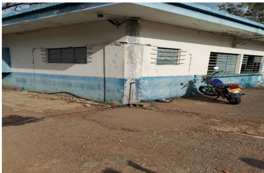
Figure 3 Cracks at Baie du Tombeau Police Station
