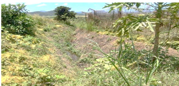
Figure 13 Stormwater drains uncleaned
