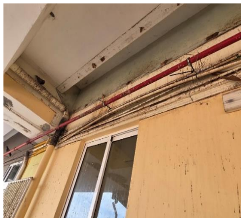
Figure 4 First floor very dirty with pigeon droppings
