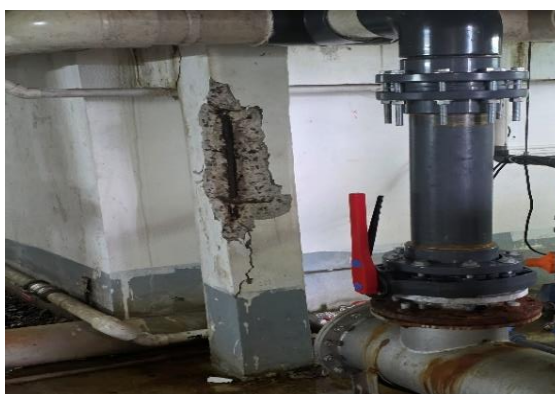
Figure 12 Cracking concrete pole
