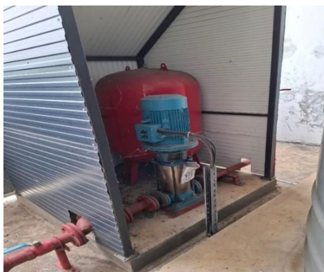
Figure 1 Pump not functioning
