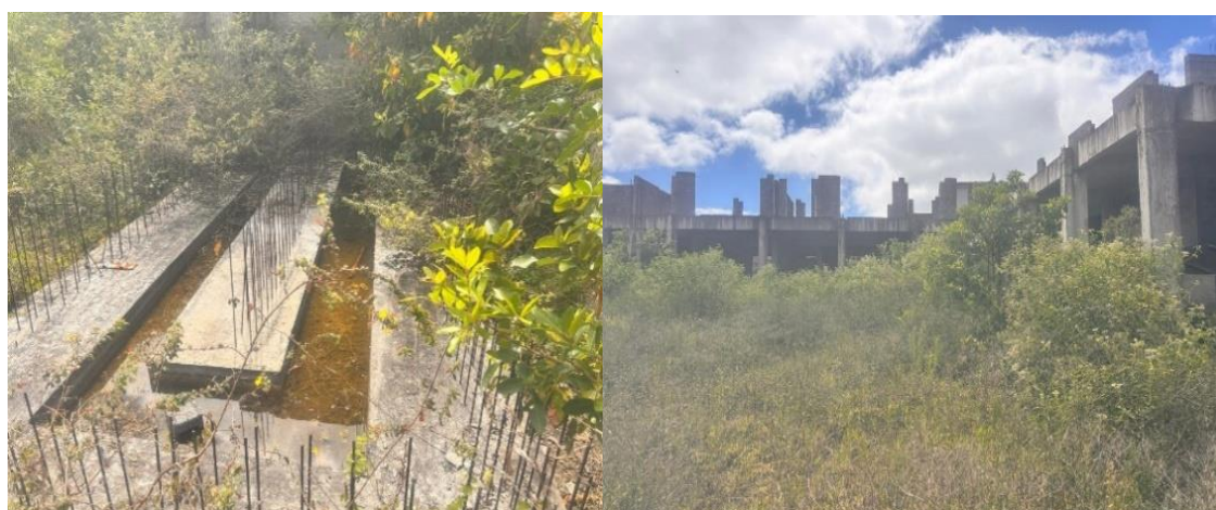
Figures 5 and 6 - Overgrown Vegetation and Rusted Iron Bars in the School Premises
