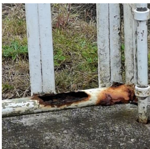
Figure 5 Rusty door on Eastern stand
